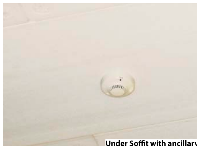
Under Soffit in Service Duct
