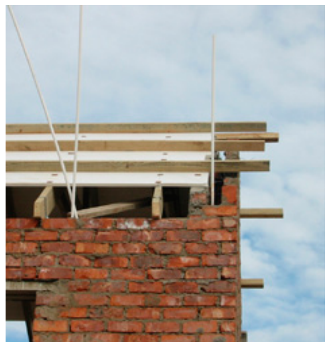
IsoBoard secured against uplift using a counter batten above, and screws and washer below
